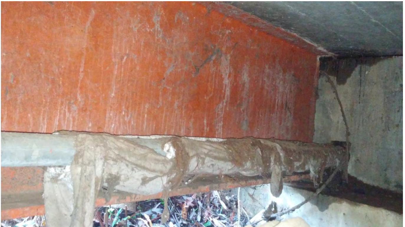
TSI (Thermal Systems Insulation) 40% Chrysotile
