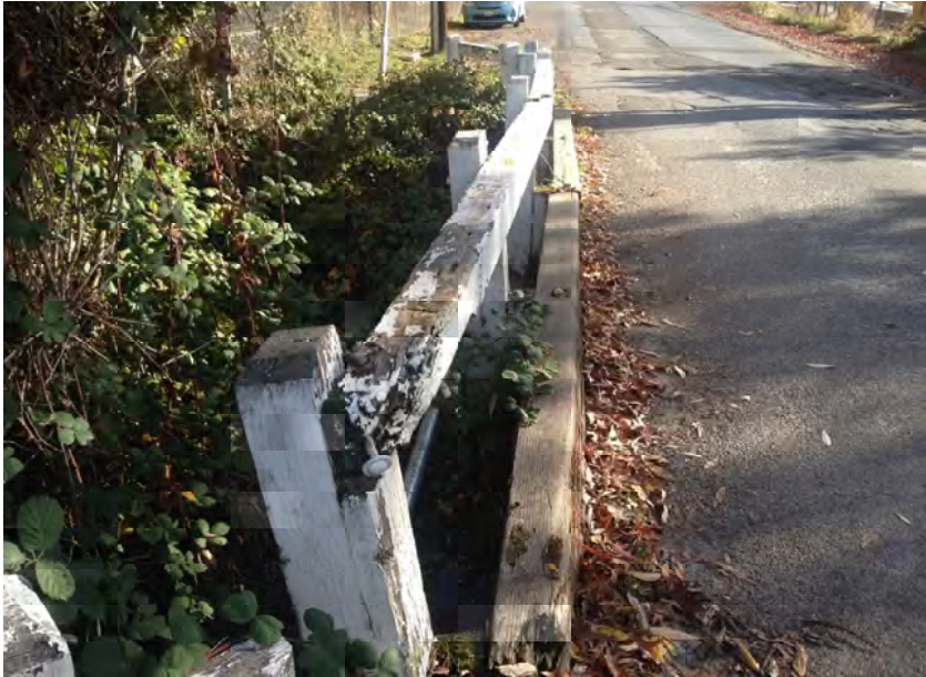
White paint on treated timber posts. Facing south from northeast corner. Taber Consultants photo 11/14/2014.
