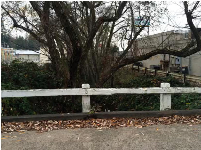
White paint on treated timber posts. Facing west from Blairs Lane centerline. Taber Consultants photo 11/14/2014.
